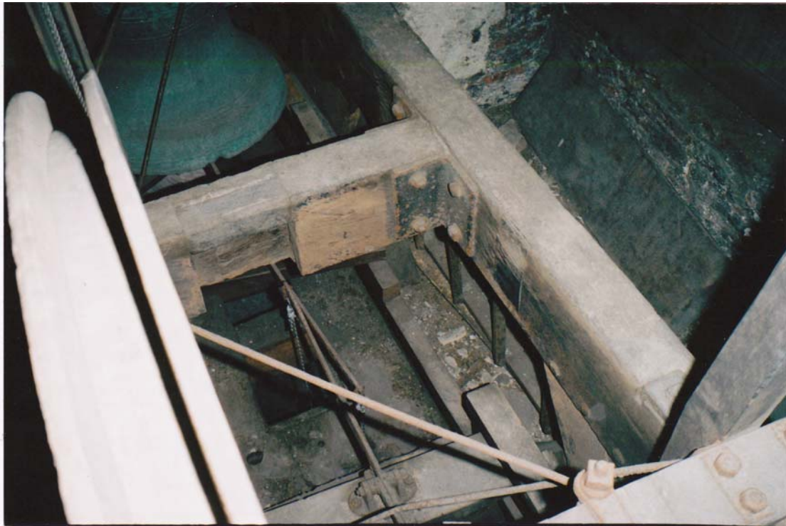
The dividing timber between the pits for the treble and second bells. The cut-off tenon shows as a dark rectangle on the side of the frame head.
