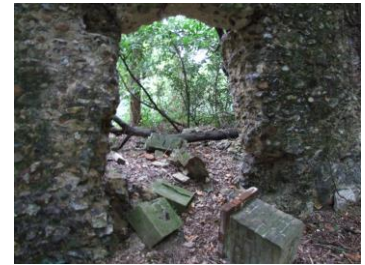
The effects of uncontrolled erosion
