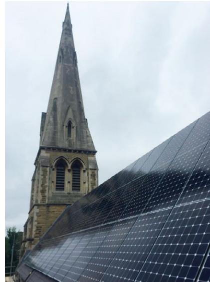
Solar Panels at St Anne's Church, Highgate © PowerUP North London
