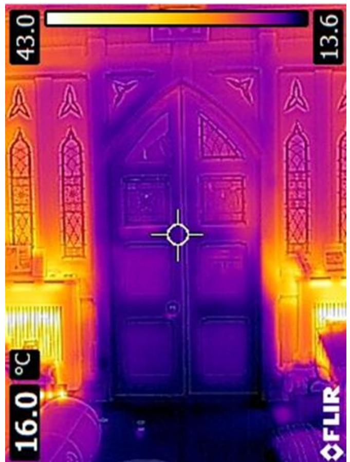
Below: Thermal image showing heat loss from cold air coming under a church door.
