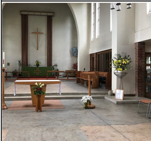
1 View of the crack in the floor that had emerged in St Edward’s, as a result of subsidence in the surrounding area.
