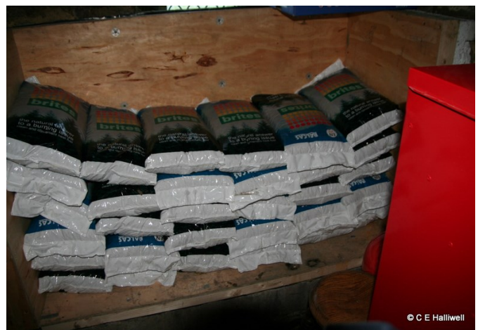
Tatham Fells, Good Shepherd Church: biomass boiler, hopper, and wood pellets
